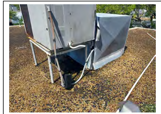
Typical AC stand and duct box
